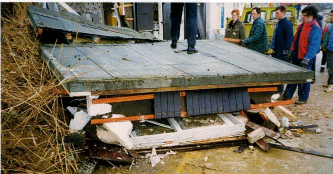
This beach cafe near Sandown, Isle of Wight was destroyed by a cliff fall. A range of stabilisation measures have been carried out following a detailed risk assessment of the cliffline.
