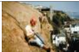
Cliff trimming to reduce risk of cliff falls, Shanklin, Isle of Wight, UK
